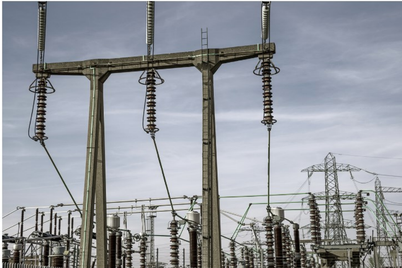
Electricity substation and cables connecting with overhead power lines (pic credit: Robert Brook/Getty Images)
